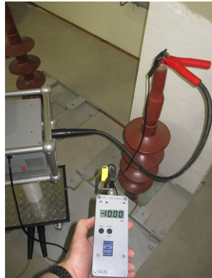
Figure 5: CAL1B connected to an MV cable (on-site)
